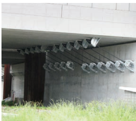
Bridge Collapse Prevention device
