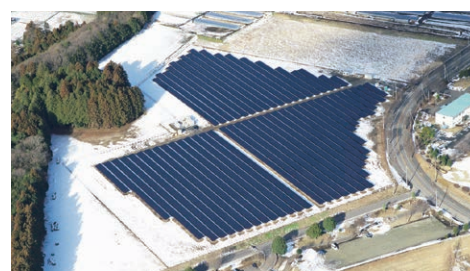
Solar power generation (Otagawa solar farm, Tochigi)
