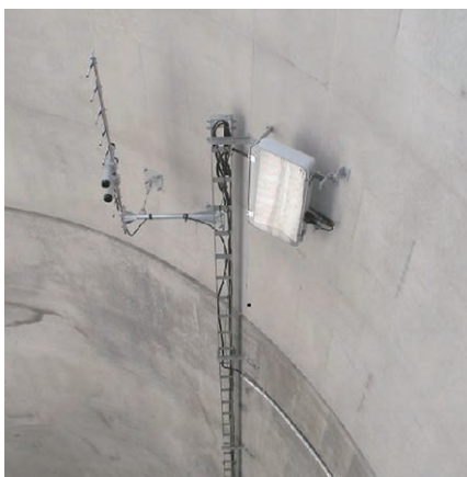
Tunnel Illumination Lamps
